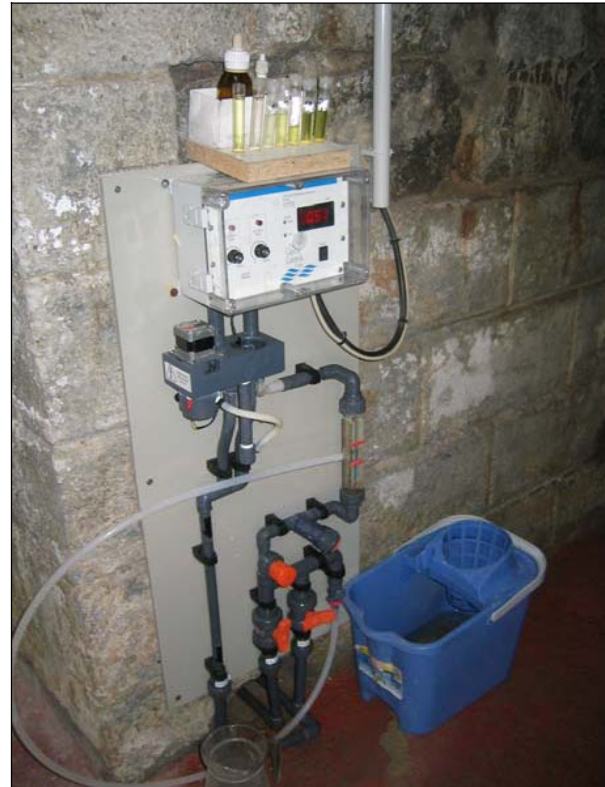
IMESURADOR CLOR RESIDUAL
